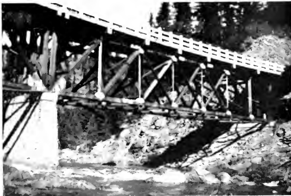
Timber bridge on Feather River Highway showing new concrete bearing blocks on truss members
